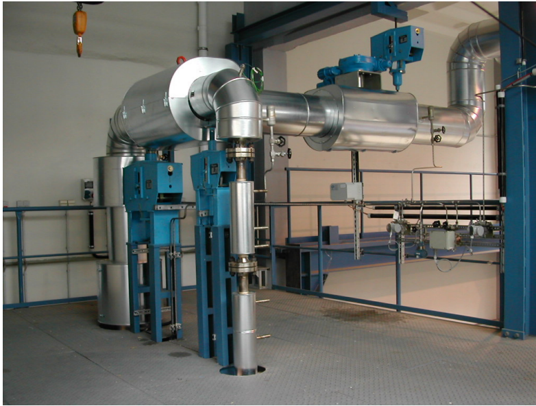
Fig. 2.5 Upper end of the vertical test sections with a part of the connecting pipe towards the steam drum
