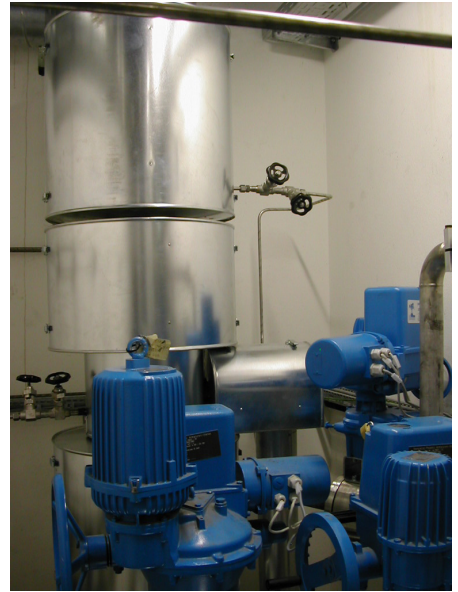
Fig. 2.6 Valves and piping at the steam injector of the large vertical test pipe DN200
