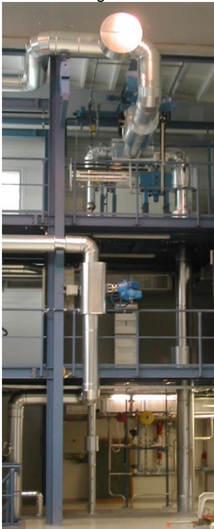
Fig. 2.4 Vertical test sections DN50 (left) and DN200 (right) in the TOPFLOW hall
