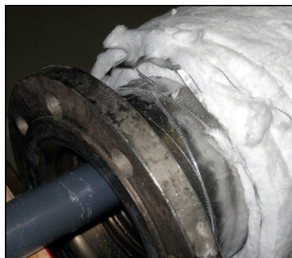
Fig. 2.12 Insulation of a hose with Superwool blanket
